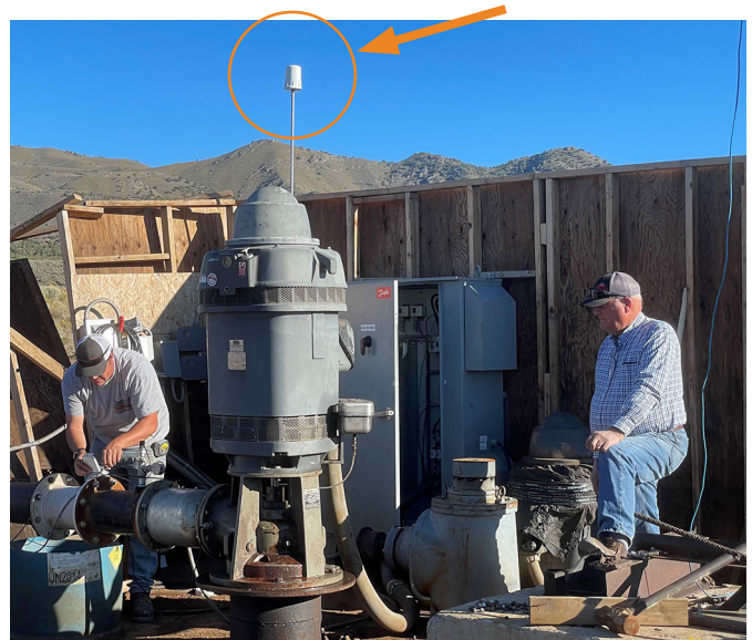
On this multi-generational farm, Marc's dad is making sure he gets the repair right. He, too, appreciates the benefits of the RANGER and the SignalFire Cloud. This is pump house #2 that a second RANGER is monitoring.
