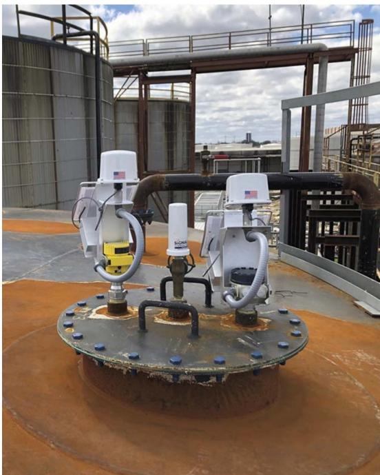
Figure 2. For easier installation, a custom-fabricated mounting bracket assembly supports the HART nodes and solar panel to provide the required power to the temperature sensor. The nodes gather data from the sensors and wirelessly transmit it to a gateway for download into an inventory software system.
