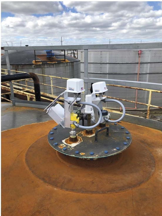
Figure 1. A configuration of HART nodes with a solar panel system installed on top of one of the terminals.
